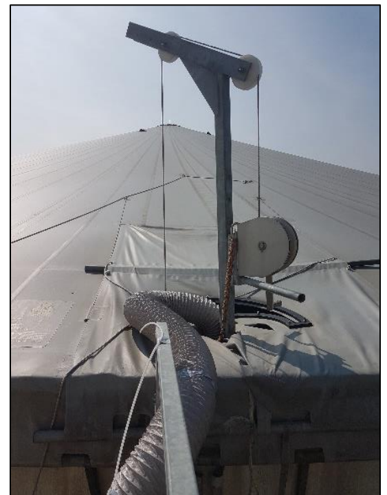
Figure 2: Measurement of the methane concentration from a not aashtigt diagestate storage tank
